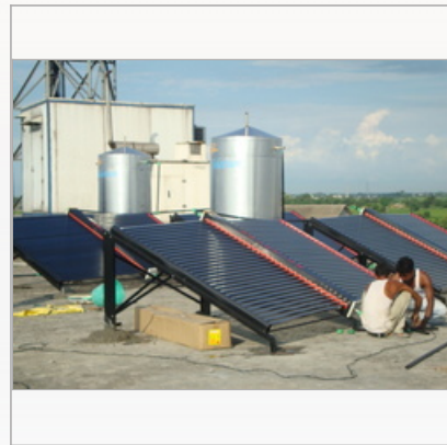
Solar Water Heater
