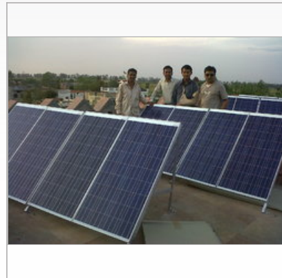
Solar Power Plant
