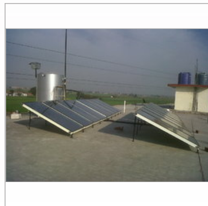
Solar Water Heater FPC
