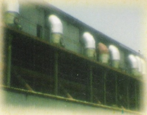
BATTERY OF CONDENSERS MULTI JET FOR SUGAR PLANT 5000 TCD
