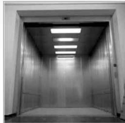
Goods, Passenger Lifts
