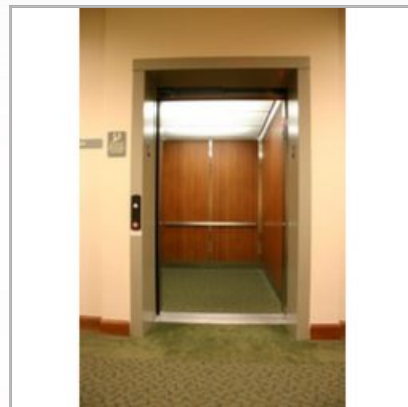
Passenger Lift And Casual Lift
