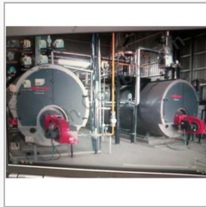
Burners And Boilers
