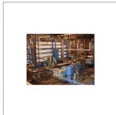
High Pressure Pump for R.O.
